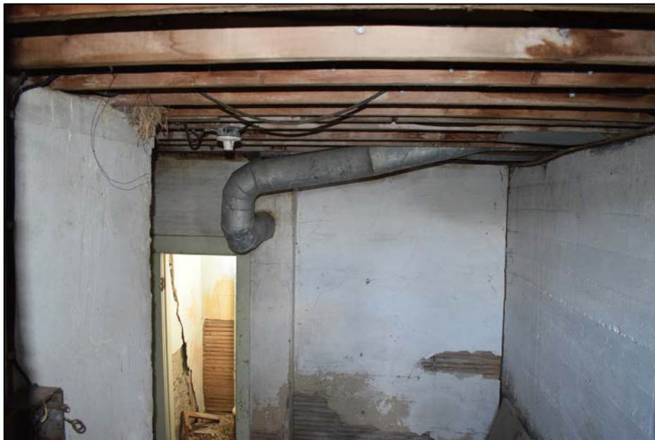
Figure 37. Ductwork in basement, doorway to boys' toilet pictured, facing south.
