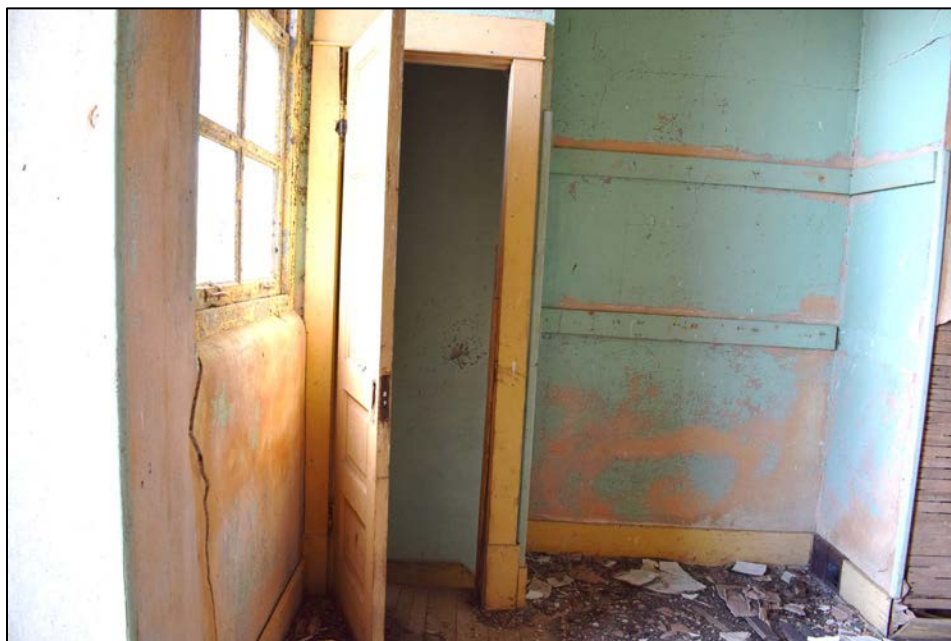
Figure 20. Inside QCRS-MC2A front door showing doorway to girls' toilet stairway, facing south.
