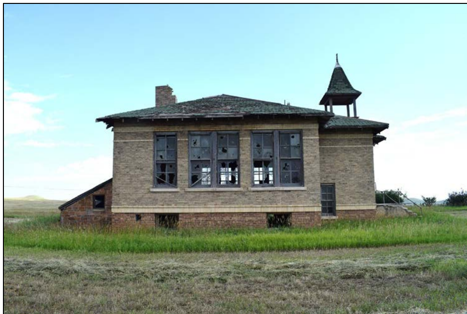
Figure 3. View of south side of QCRS-MC2A facing north.
