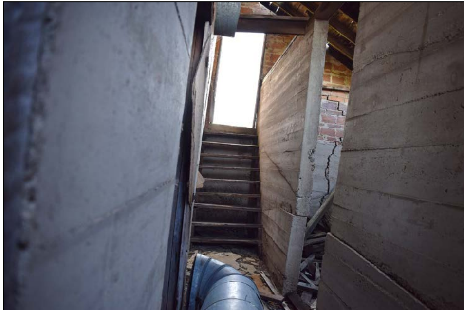
Figure 46. Addition on rear of building, photo taken from doorway in basement facing south.
