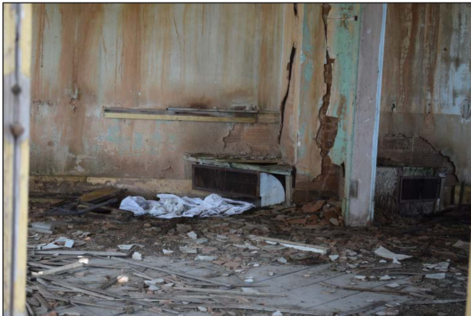
Figure 33. Forced air registers on center of rear wall facing west.
