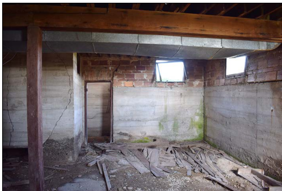
Figure 42. At base of stairs into basement, facing west, doorway pictured leads to rear addition.
