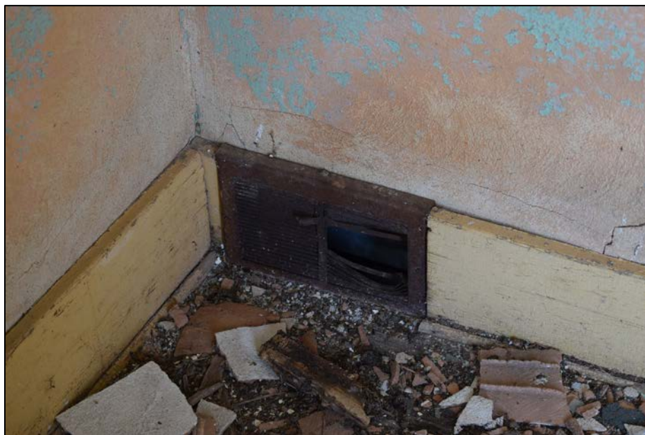
Figure 34. Forced air register in vestibule, interior wall between vestibule and classroom, south side of QCRS-MC2A.
