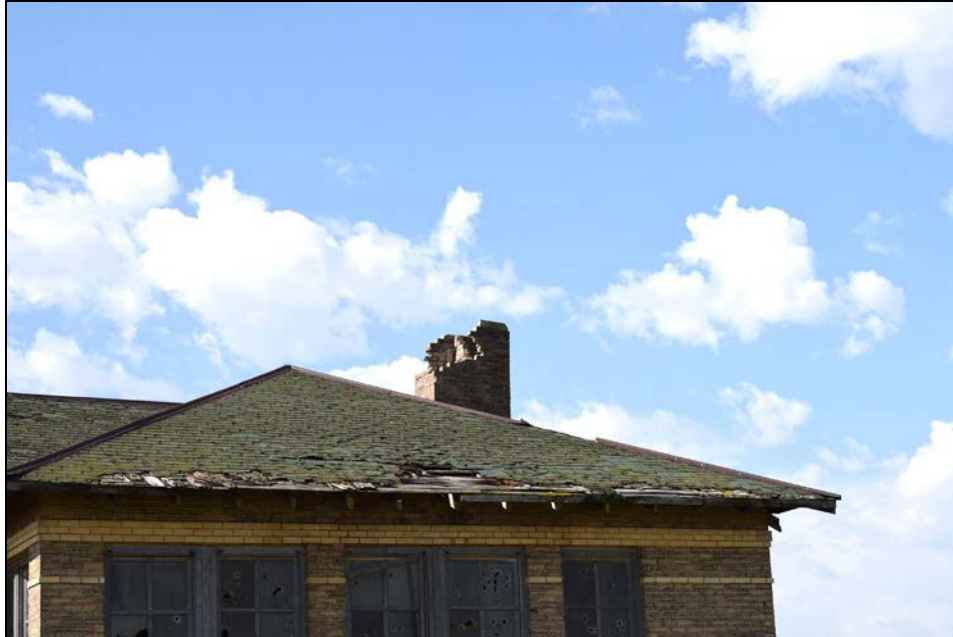
Figure 17. Detail of roof line and chimney on rear of QCRS-MC2A facing southwest.
