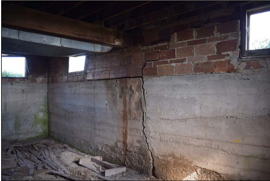
Figure 47. North basement wall showing bowed foundation.
