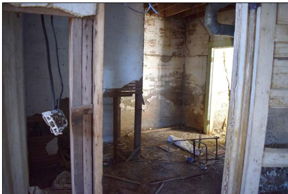
Figure 38. Entrance to room in basement along east wall, doorway to boys' toilet in background.
