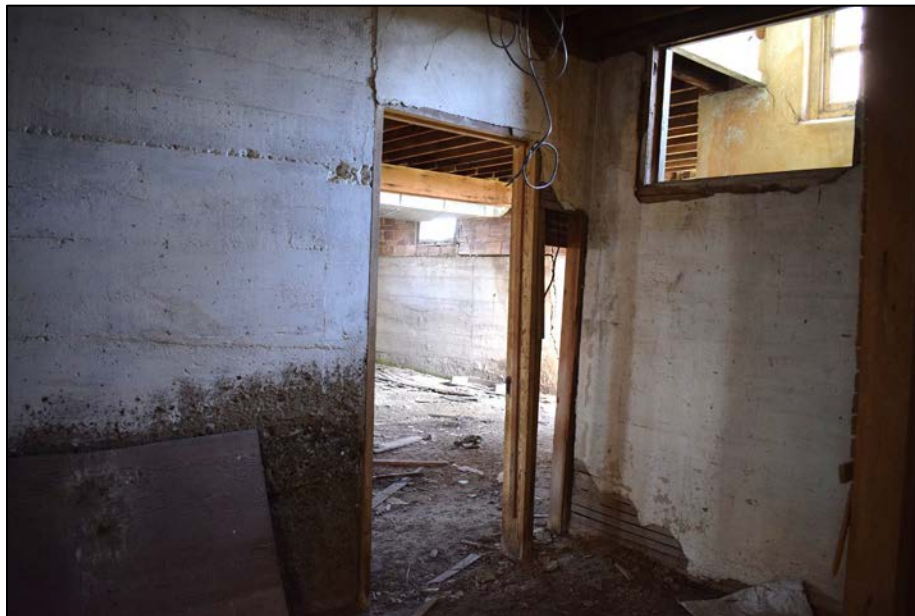
Figure 41. Doorway into basement room along eastern side of building. Interior stairwell window also visible, facing northwest.
