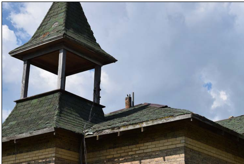
Figure 15. Detail of roof elements and vent behind bell tower on QCRS-MC2A facing southwest.
