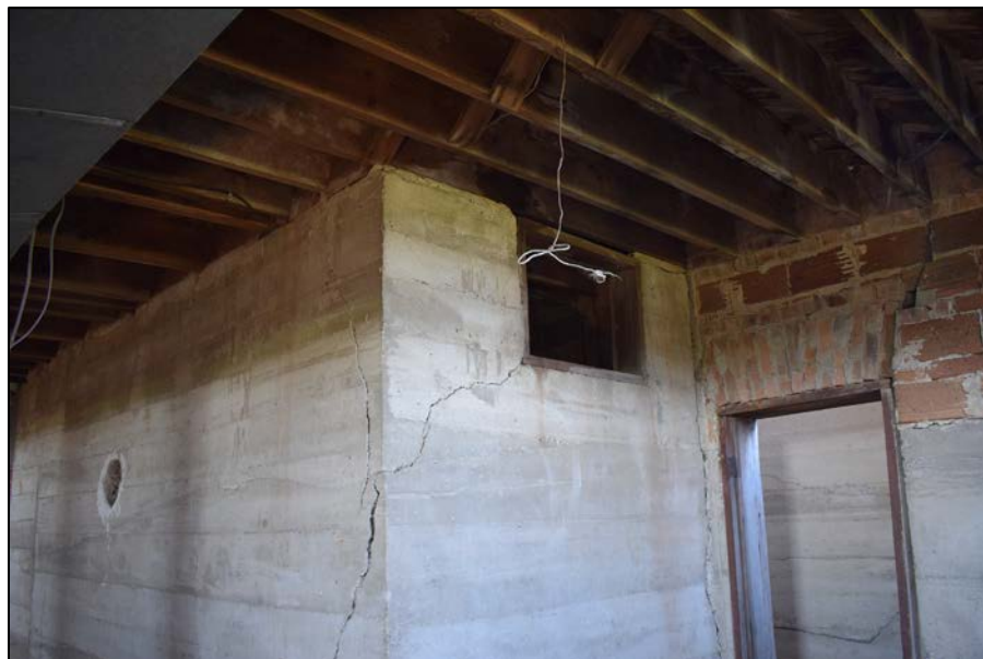
Figure 44. Detail of first floor supports as they rest on basement foundation, rear of building facing southwest.
