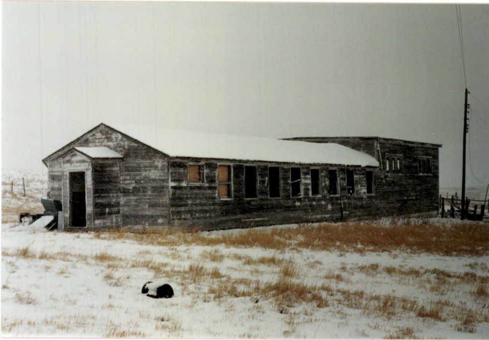
Feature 1, north and west elevations, view to the southeast; 970919c, Roll 100, Negative 18.
