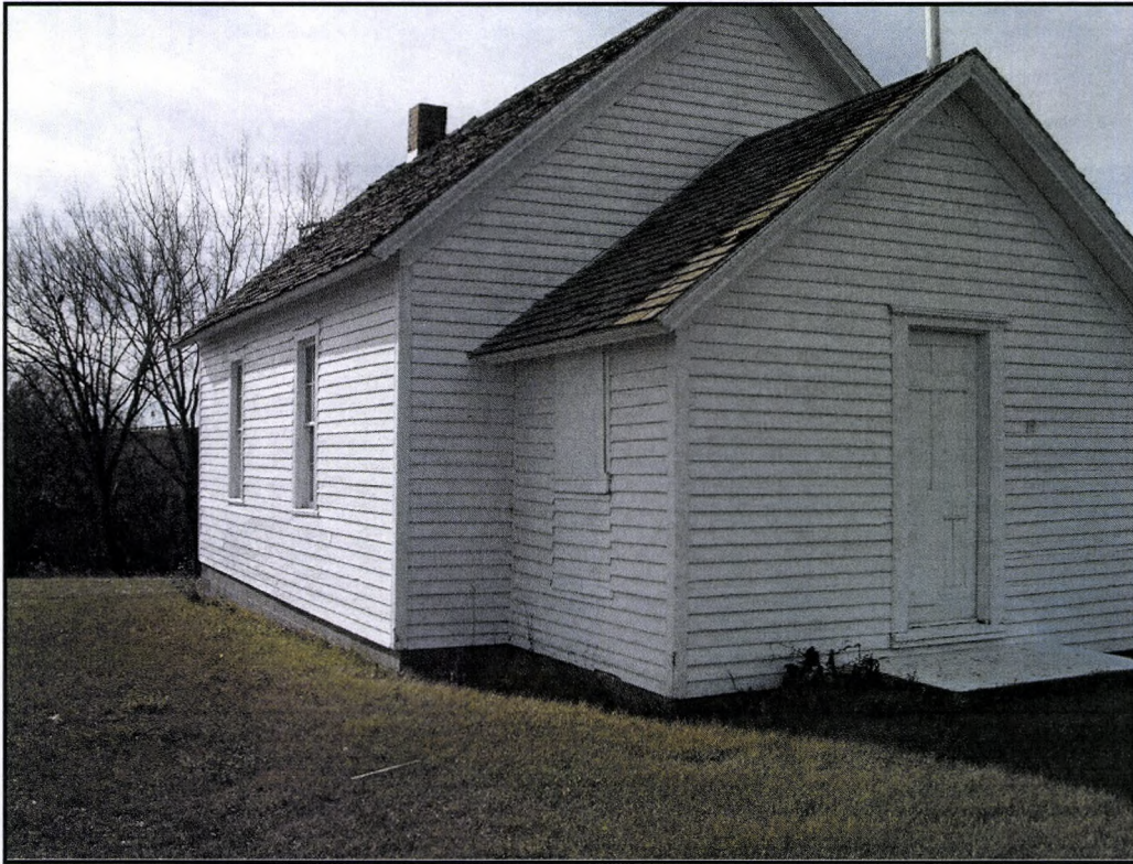
Figure 7: Overview of the northeastern corner of the Nettle Creek School, view to the southwest.
