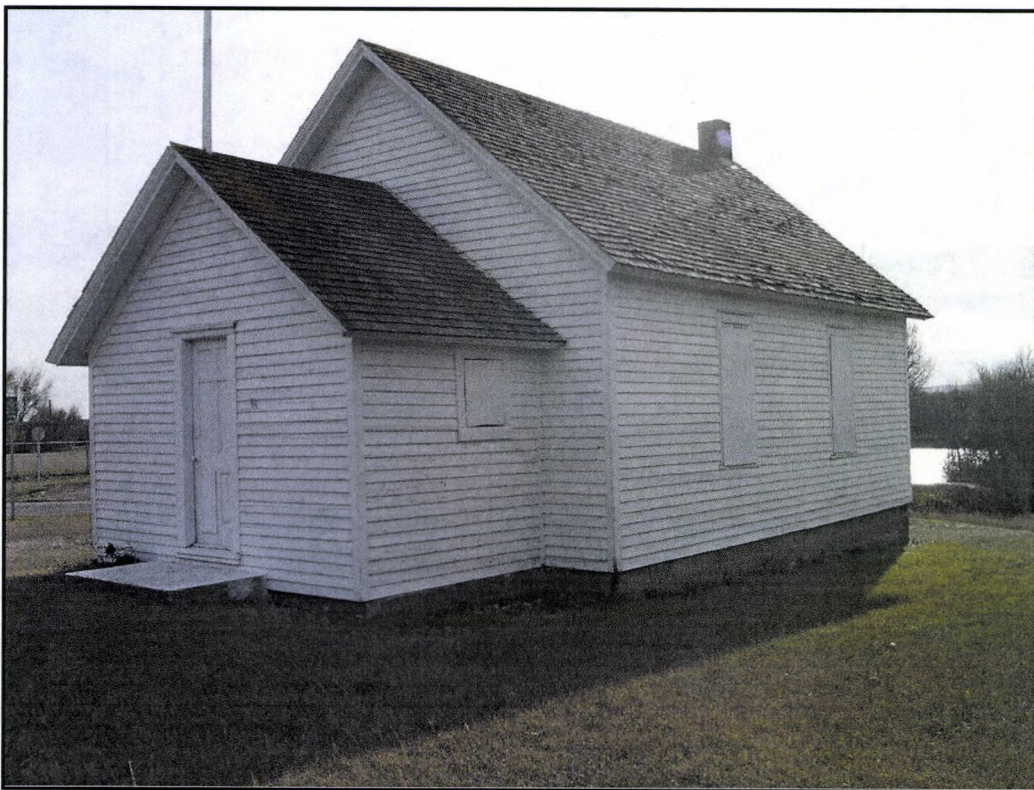
Figure 6: Close up of the northwest side of the Nettle Creek School House, view to the south-southwest.
