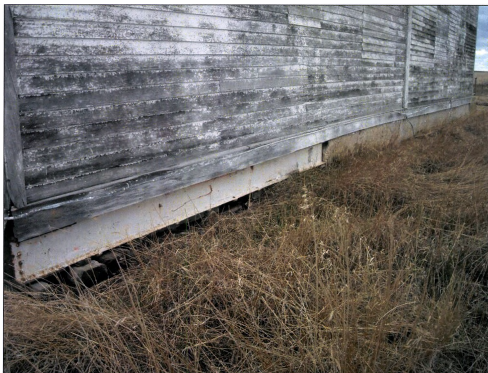
Figure 8. 32MN831, detail view of foundation on west side of Feature 1, facing southeast.
