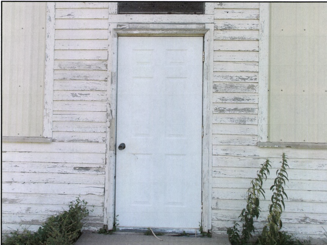
Figure 11: Close up of the main entrance (east side) showing that the door appears to have been painted or replaced recently, and two replaced windows.
