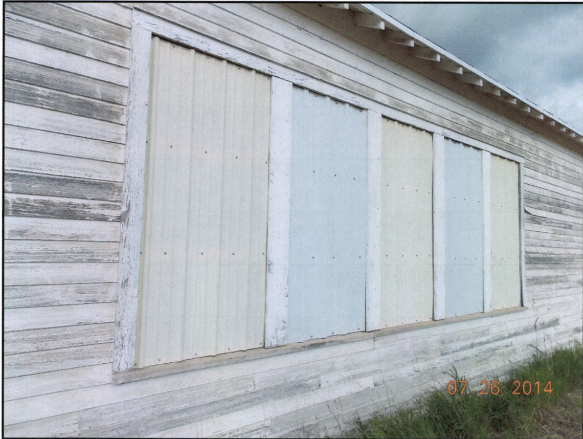
Figure 8: Close up of the south wall and the five windows, now containing sheet metal, that form one continuous portal.
