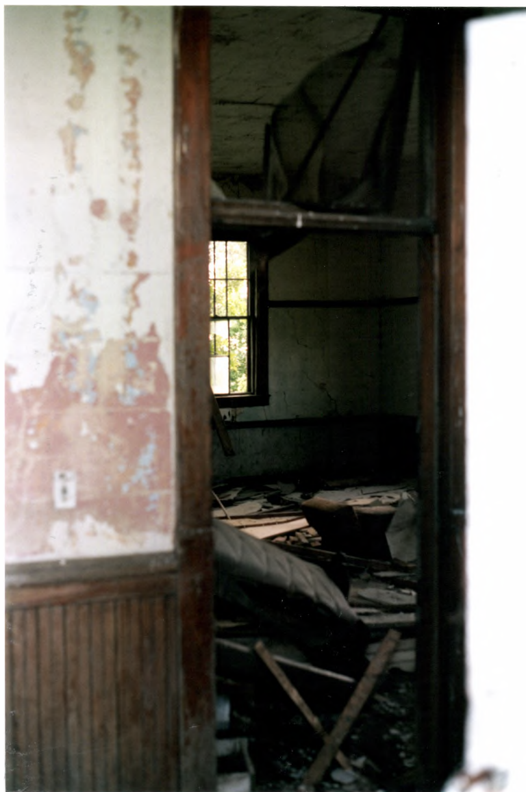
Feature # 1, north room viewed through entry vestibule and doorway in southeast corner of room, roll 1, frame 28.
