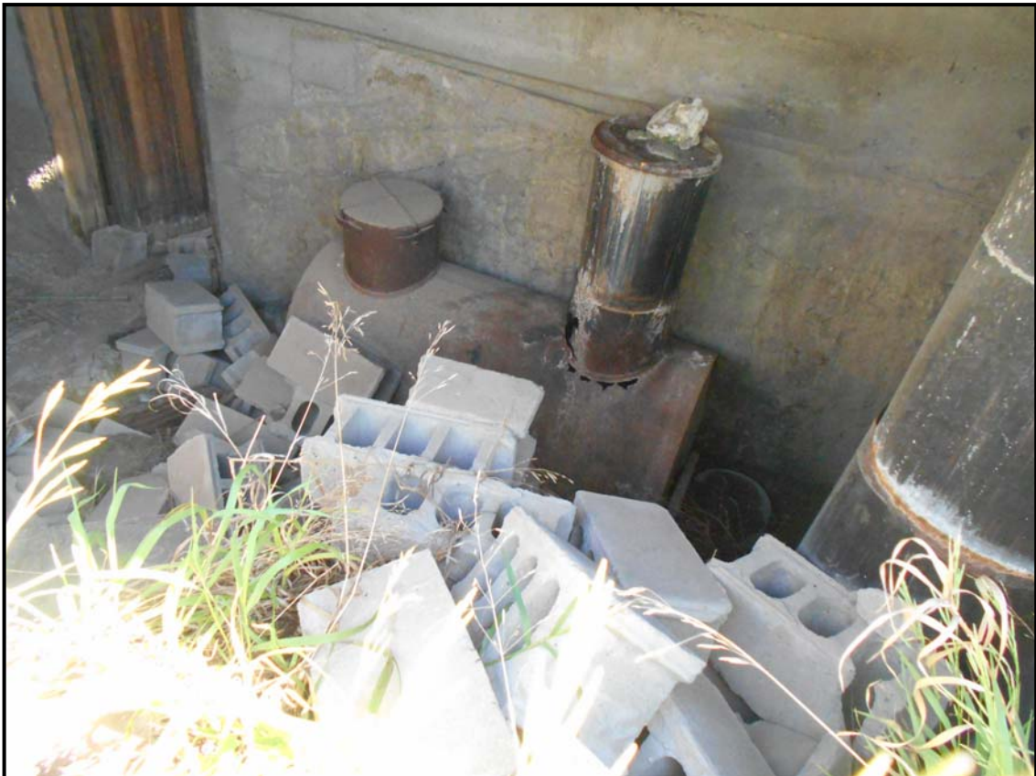
Figure 9: Overview of the boiler in Feature 1.
