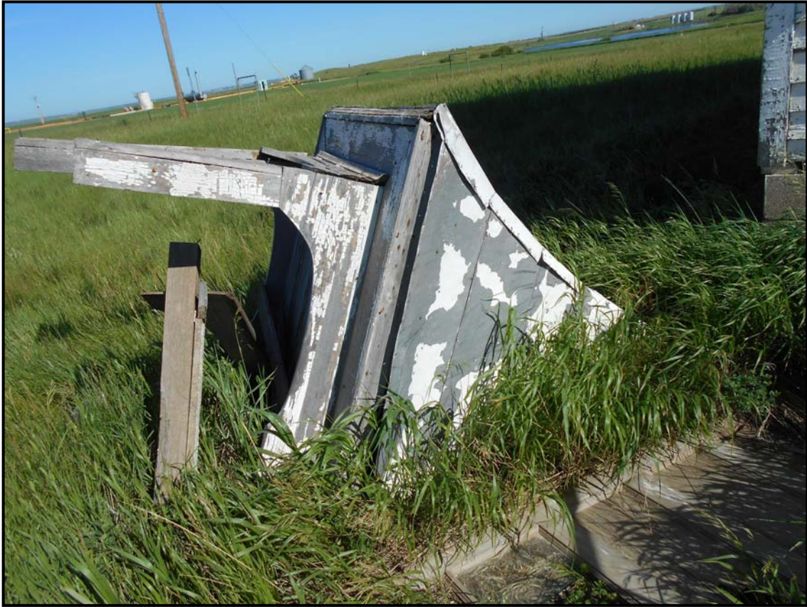
Figure 10: Close up of the fallen cupola next to Feature 1.
